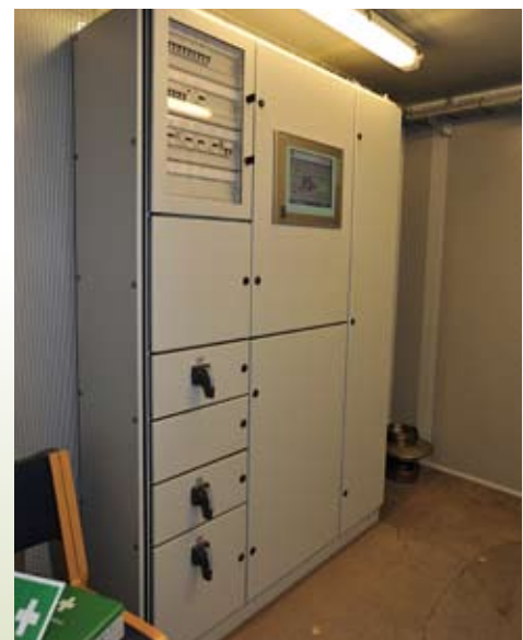
A pared-down control panel
